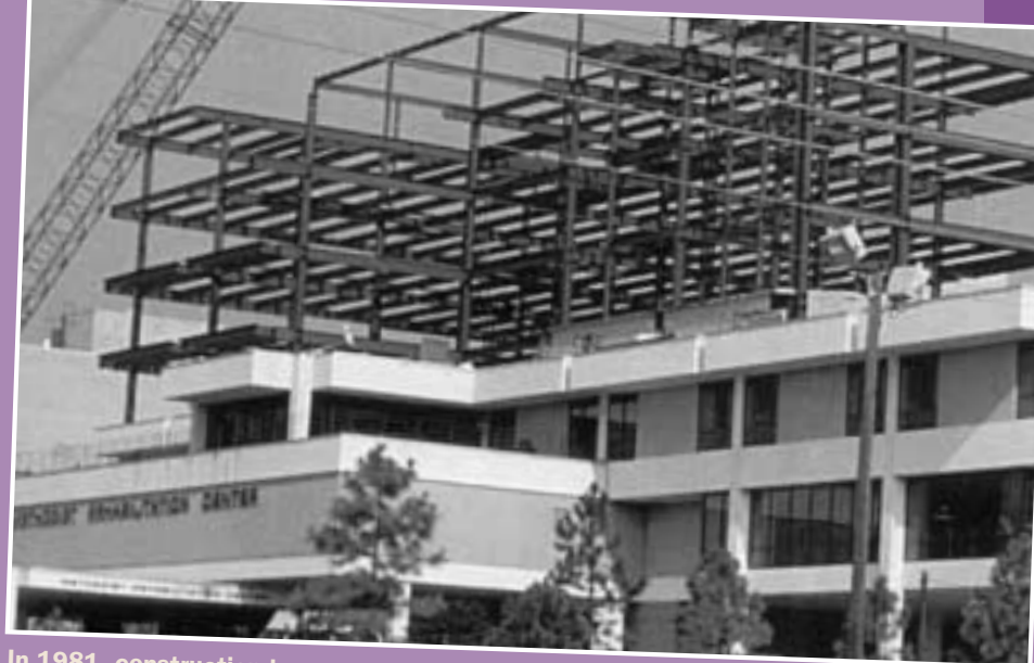
In 1981, construction began on an additional four hospital floors, expanding the facility’s capacity from 60 to 124 beds.
